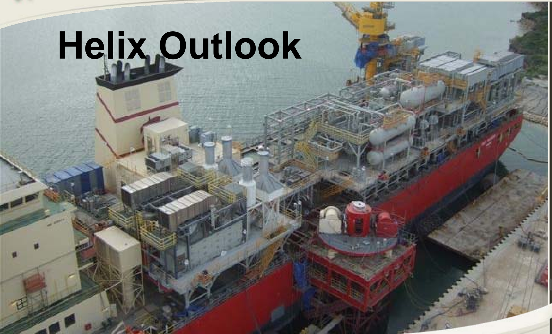
Helix Producer 1 topside module installation progress at Kiewit Offshore Services fabrication yard
