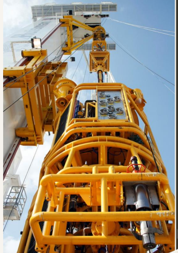
Subsea Intervention Lubricator system onboard Well Enhancer
