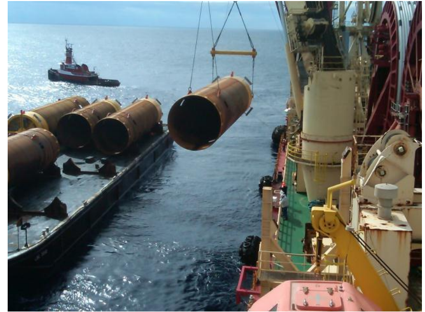
Express installing suction piles in the Walker Ridge block of the Gulf of Mexico
