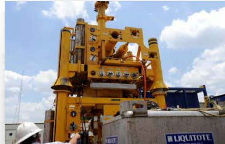
Intervention Riser System
