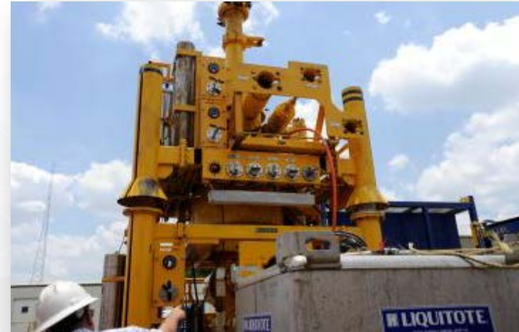
Intervention Riser System
