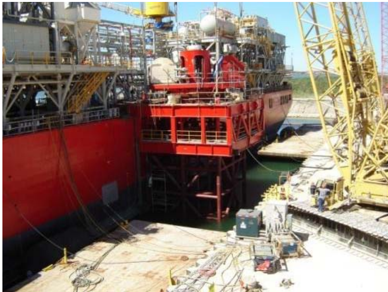
Disconnectable Transfer System
