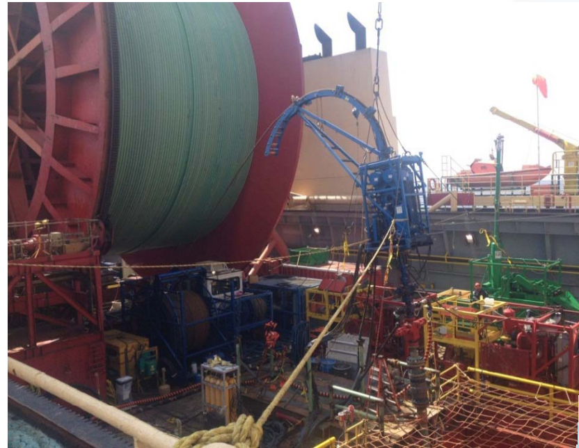
Coiled tubing connected to the pipeline recovered through the moonpool of the Express
