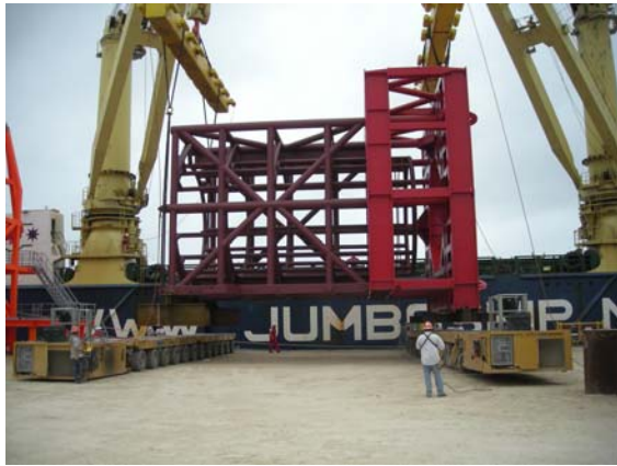
Offloading of the HPI DTS Hang-Off Structure at Kiewit's yard, Ingleside Texas
